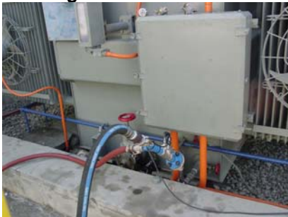
Suction Line Connection to Plant
