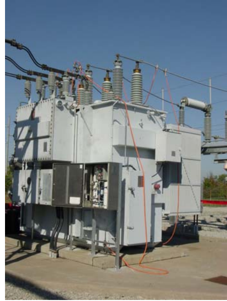
Installation at Canadian Niagara Power - 60 MVA Transformer
