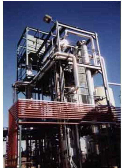
Installation at customer site
